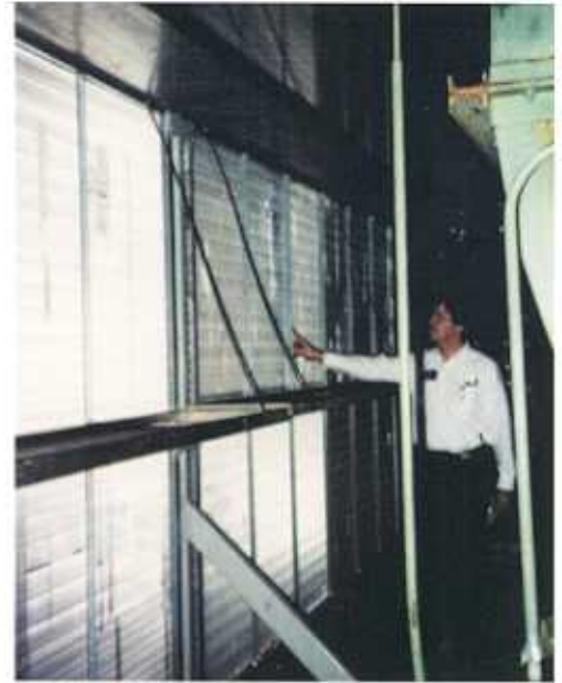
An interior view of the newly installed chilled water coils with Tom Cronin, chief engineer, Sears Tower The John Buck Company.
