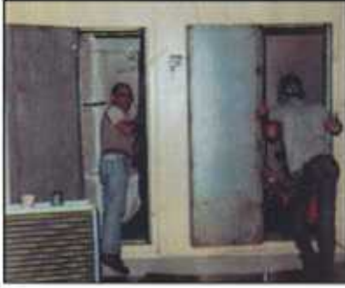
Workers begin the replacement process by removing old coils from the hospital's air handlers. The requirement for close tolerance is exemplified by the small opening of the entry doors.
