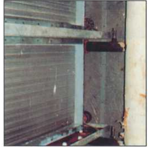
Another example of Heatcraft's quality replacement coils is demonstrated here. Because the air handlers were built around the original coils, replacement was extremely difficult due to the lack of room.
