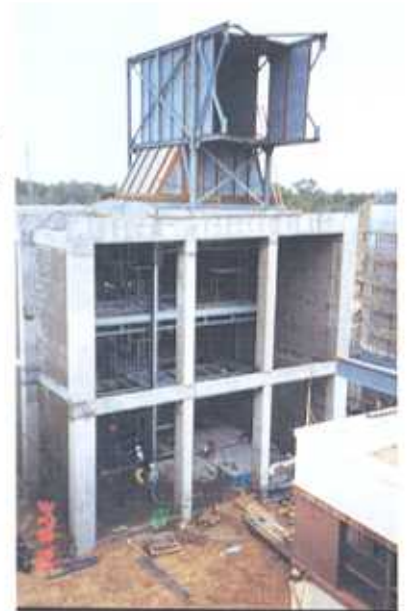
This building will house the 84 custom made Heatcraft coils for the environmental chamber.
