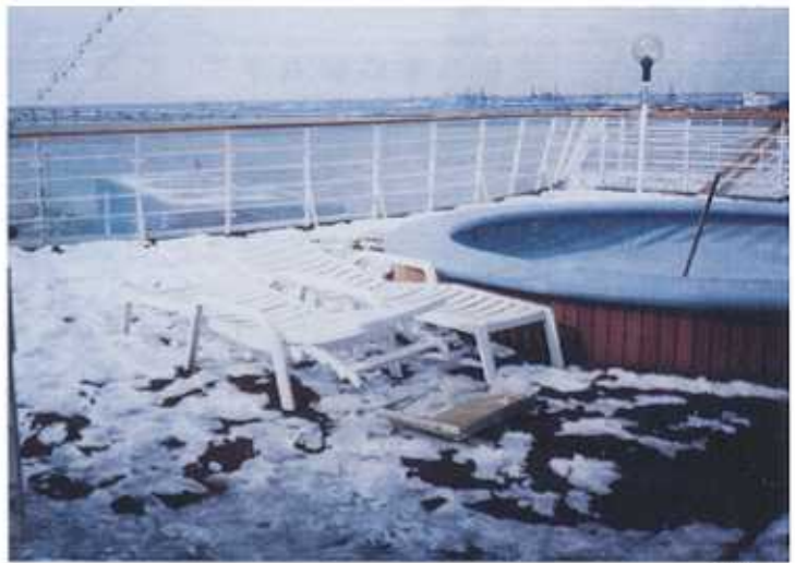
While the ships were dry-docked, unusually cold weather iced over the decks and froze the old cooling coils.
